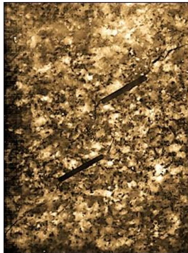
HSV Frame: Sketch 9 showing visible cracking
